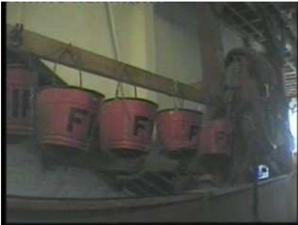
Fire buckets filled with sand
